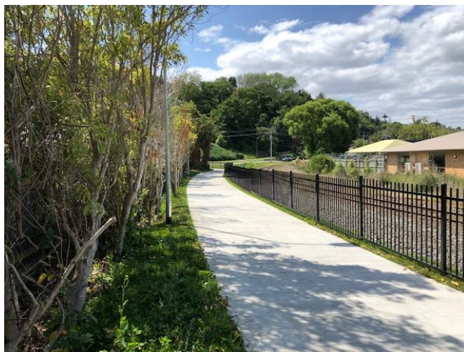
Photo: Completed Te Tuaiwi shared pathway located in Kiwirail corridor between Glasgow Street and SH3.
